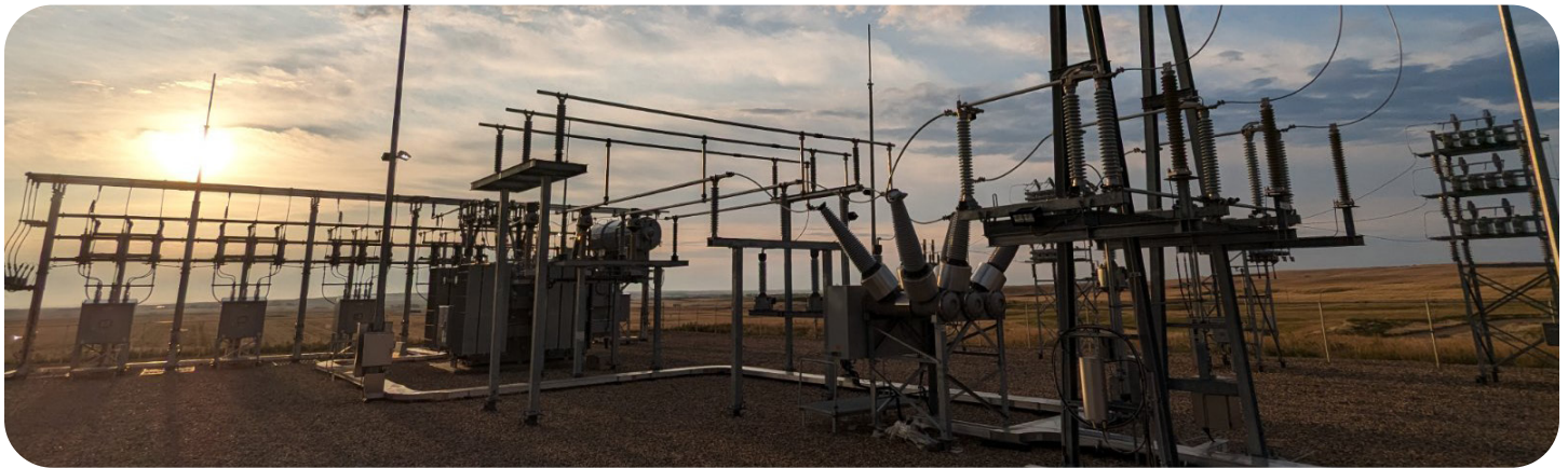
Figure 1: Substation in Hand Hills Wind Facility
